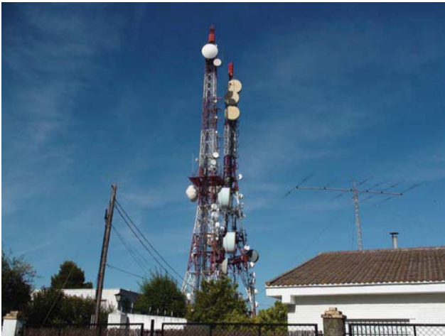
Fig. 2. Valencina broadcasting center transmission towers
